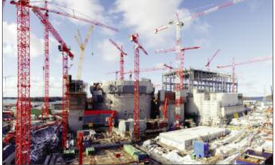
Olkiluoto 3 is under construction in Finland. The reactor is expected to go on line in 2011.
